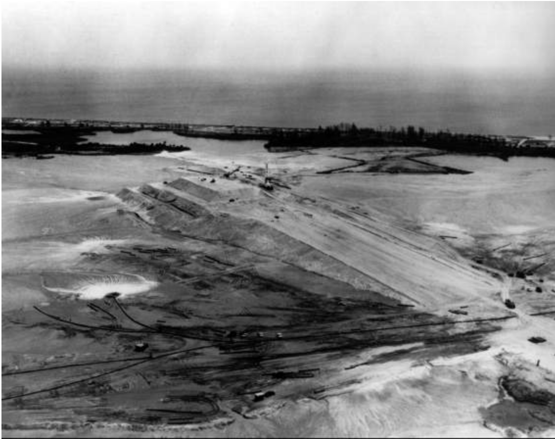
One of the big sandpiles: hydraulic fill piled on the site of LC-39, pad A, June 1963.
