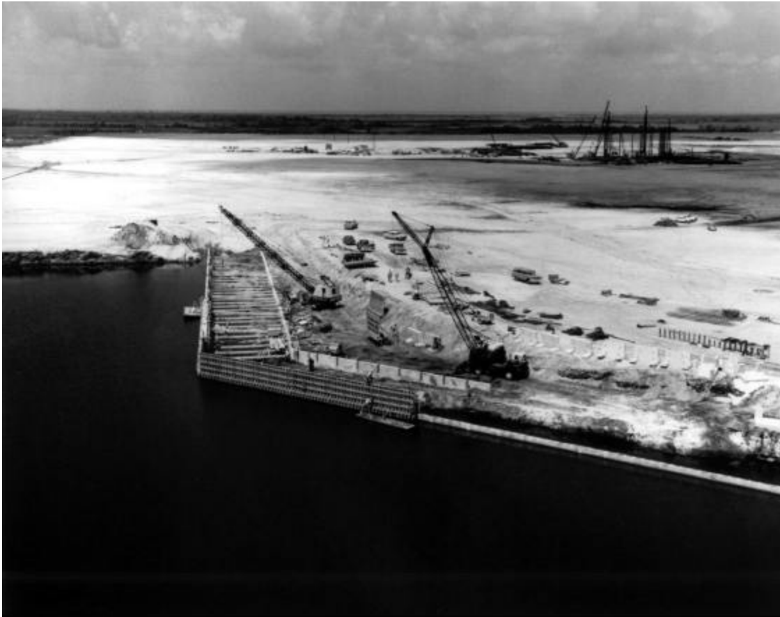
The wharf under construction at the turning basin, with assembly building site in background, August 1963.
